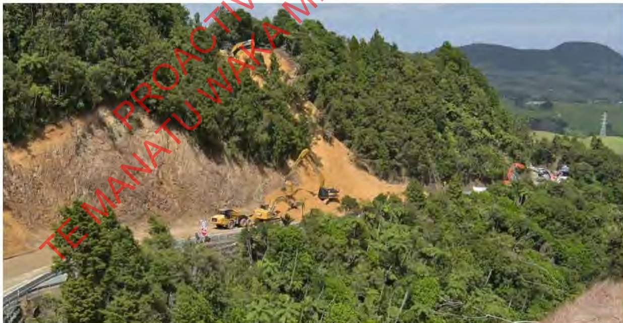
Cutting material and vegetation clearance at sites D, E and F (Continued next page)
