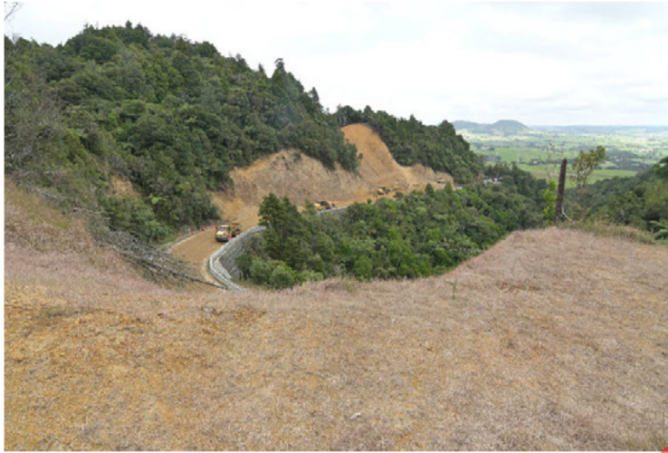
Photos 3 and 4: Cut site near waterfall corner (site E) showing a distance and a close-up view taken mid-March. The close-up view shows the extent that excavated dirt from the hillside covers the road where traffic would normally be.
