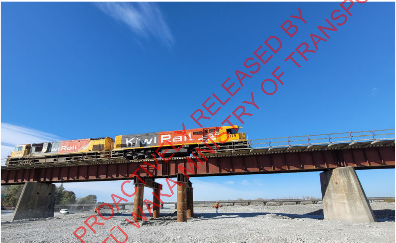
Caption: test train runs on the Rangitata River rail bridge on 25 April 2024.
