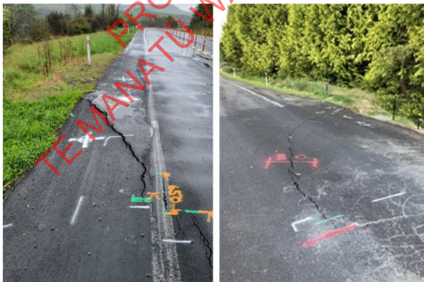
Cracking due to ground movement
